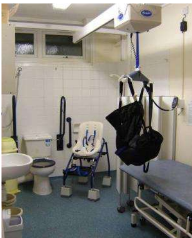
Care room with electric overhead tracking hoist
